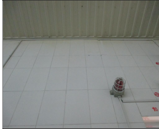
Photo of fire safety equipment Fire alarm.JPG
