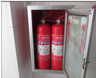
Photo of fire safety equipment Fire extinguisher.JPG
