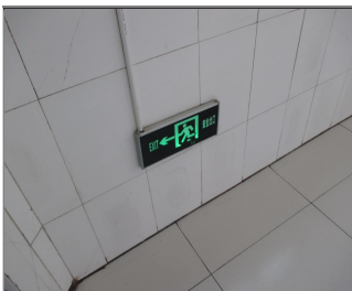
Photo of fire safety equipment Escape sign.JPG
